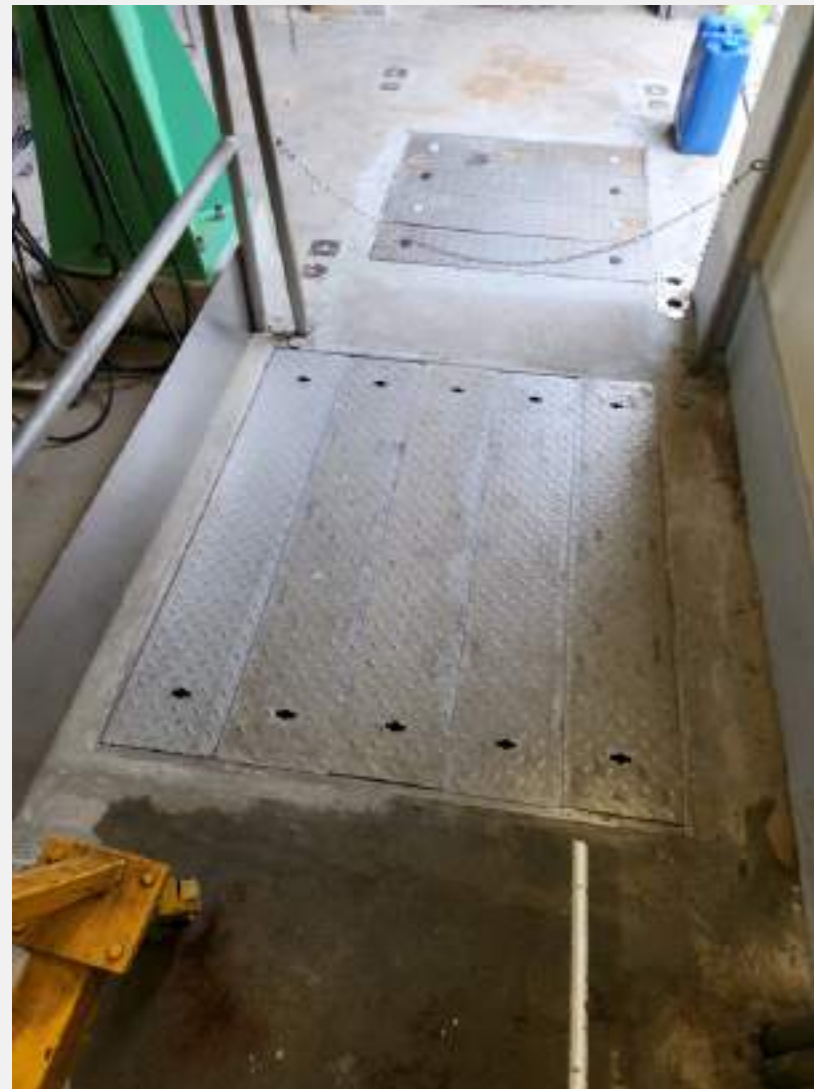
Example: Floor Opening
